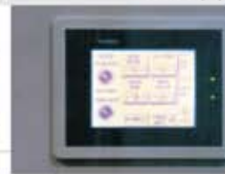
Control system with LCD screen display
